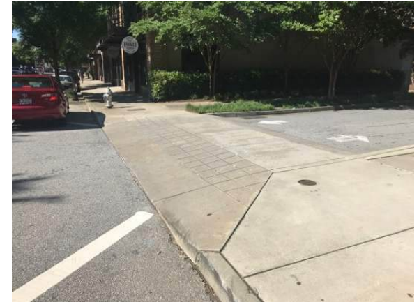
Figure 7-1: At private drives and Accessways, slope curb cut up to sidewalk level to maintain sidewalk continuity as shown in this example.
